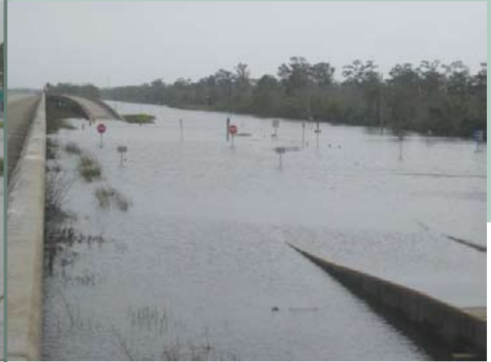
The Ruddock exit of I-55 is under water from heavy rain and high winds.
